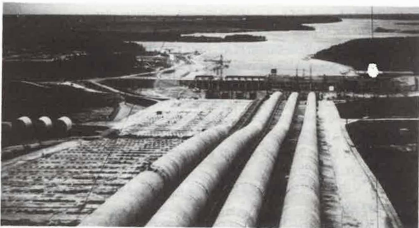
• A view of Kruonis Hydro-accumulation Station showing the construction of the fourth unit (see page 37).
